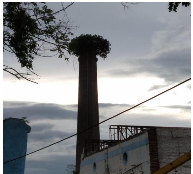
One of the red-brick boilers of the Titagarh Jute Mills No 1. The shock of shrubs atop the boiler shows that it has long fallen out of use.
